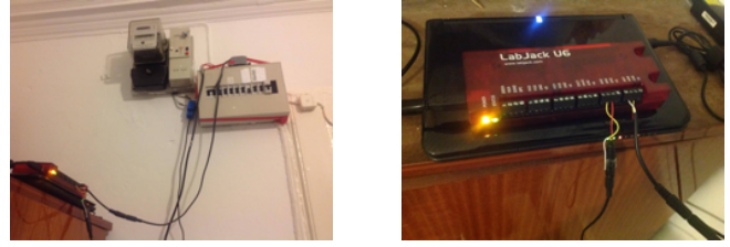
Fig. 1. Whole-house monitoring hardware installed in the main breaker box: general overview (left), DAQ system (right).
