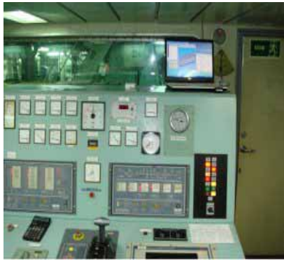
Fig. 4. Control room for main-engine
